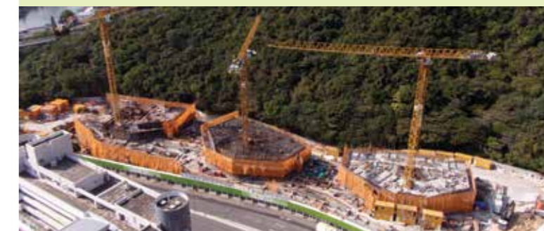
地盤內三個天秤使用節能的LED燈，以減少耗能。 Three tower cranes at the site which use energy-saving LED lighting.
