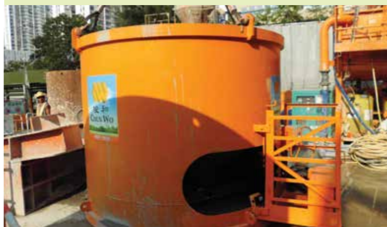
遙控混凝土載斗已廣泛推廣至俊和所有的地基項目。 The Unpiloted Concrete Skip has been widely extended to all foundation projects.
