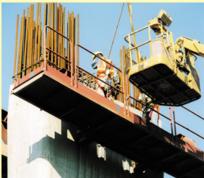
工程隊伍準備裝嵌橋身的組件。 Project team prepares for the installation of the pre-cast segments.
