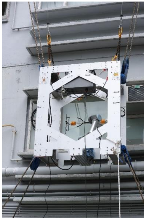
Photo2: The cable-driven robotic system has been set up outside a building on the CUHK campus to test and demonstrate it.
